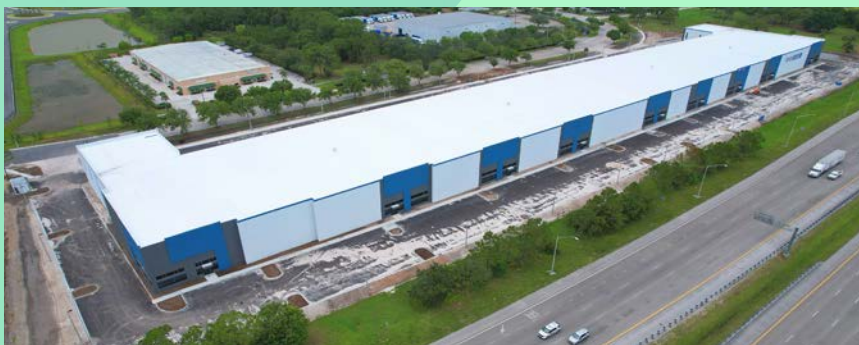
Construction was being finalized at the Interstate Commerce Center along I-95 in June.
