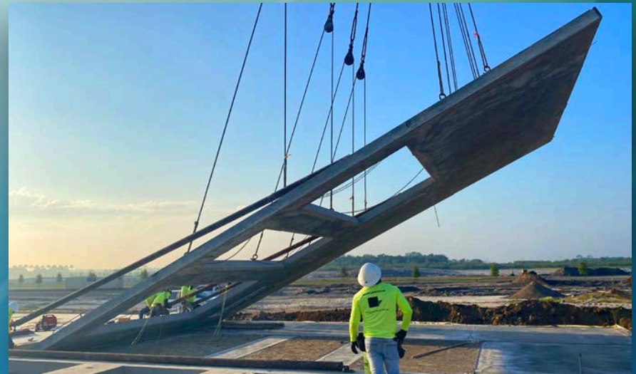
Walls went up in February for the Sansone Group's 520,000 SF spec industrial building in Legacy Park at Tradition
