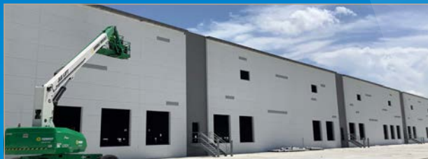
Construction on the 520,000-square-foot Class A industrial building had moved into its final stages in June.
