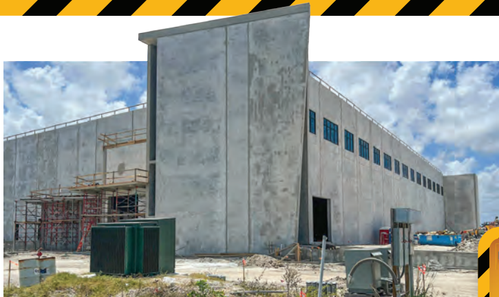
Construction is progressing on the manufacturing facility for OCULUS Surgical in the Tradition Center for Commerce.
