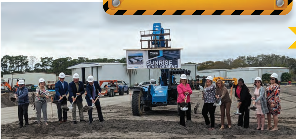
In February, APP Jet Center at Treasure Coast International Airport broke ground on 30,000 SF of new hangars and an extensive renovation of the fixed base operator's facility. Plus One Air is also planning to add a 15,600 SF hangar to its TCIA footprint.
