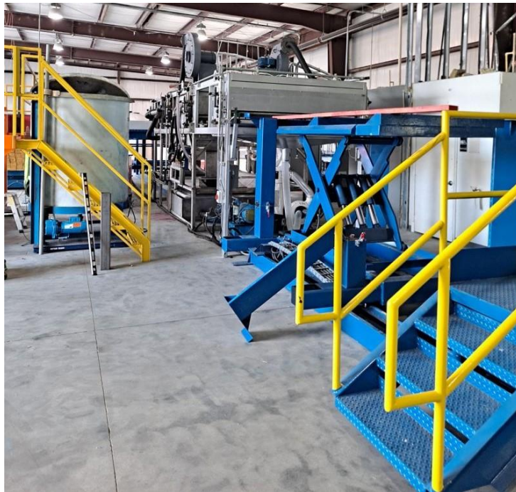
The treating line at Chemical Technologies' Techwood facility in Fort Pierce.
